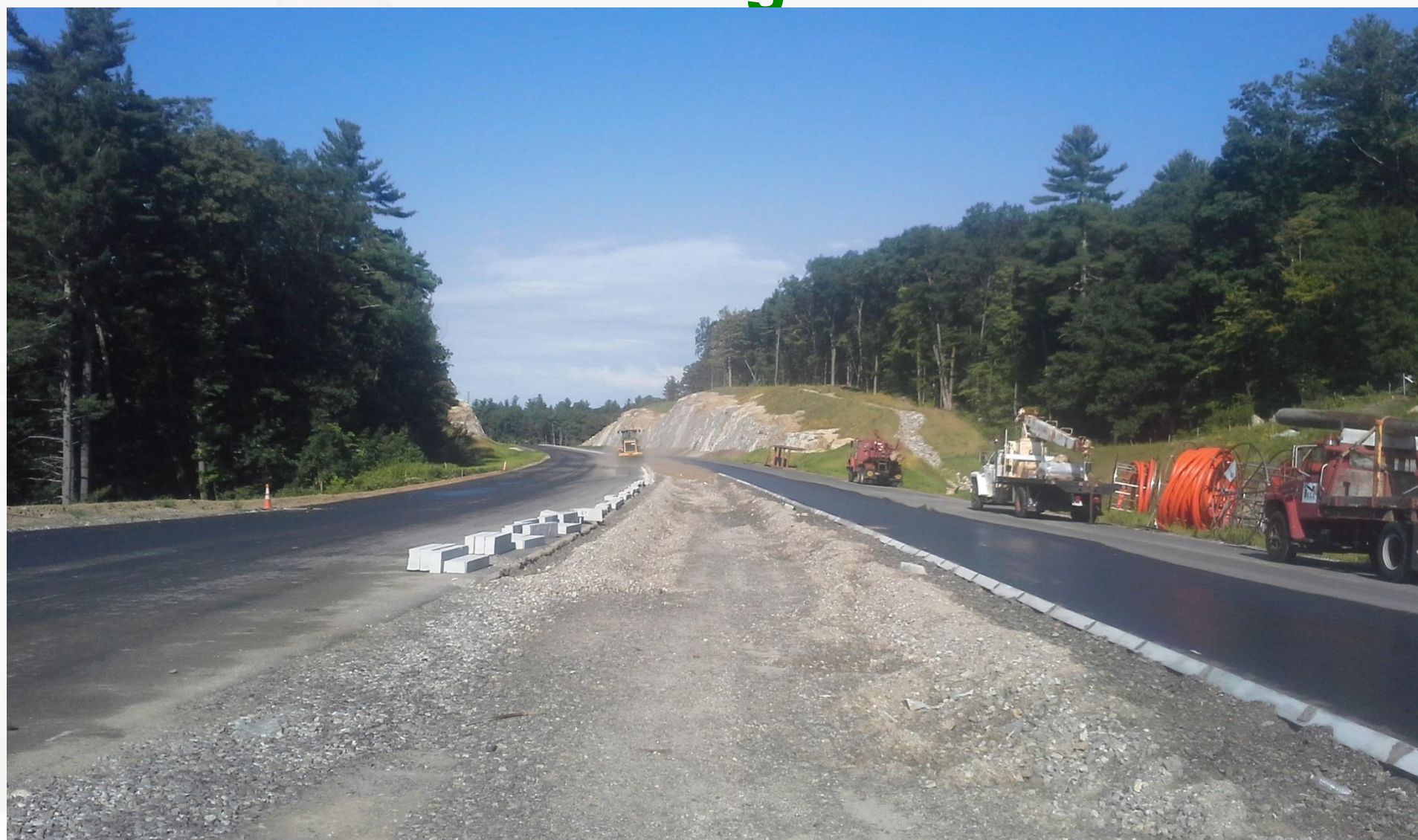
New NH Route 111 Facing West (next to the new Exit 3 SB ramps)
